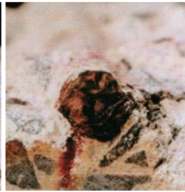
Unprotected steel surface subjected to an immersion trial.
